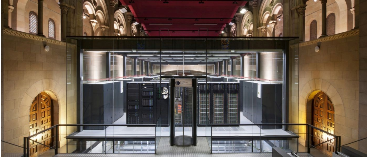
LeSI installation in the Barcelona Supercomputing Center
