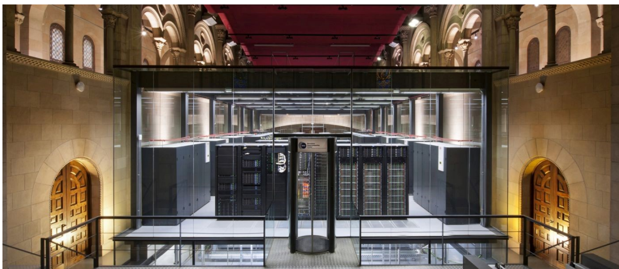
LeSI installation in the Barcelona Supercomputing Center
